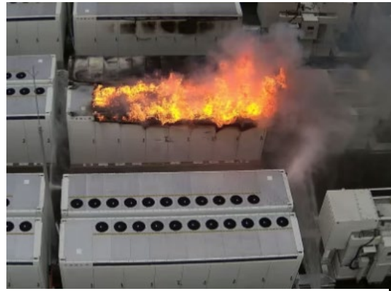
Figure 1: Lithium Ion Battery on Fire
